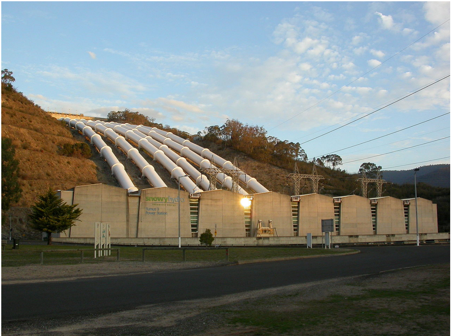
Tumut-3 Power station in the Snowy Mountains: Each penstock feeds a hydro-generator and the water is then collected in the Tumut reservoir below the turbines and pumped back up to the Talbingo Dam using off-peak electricity.
